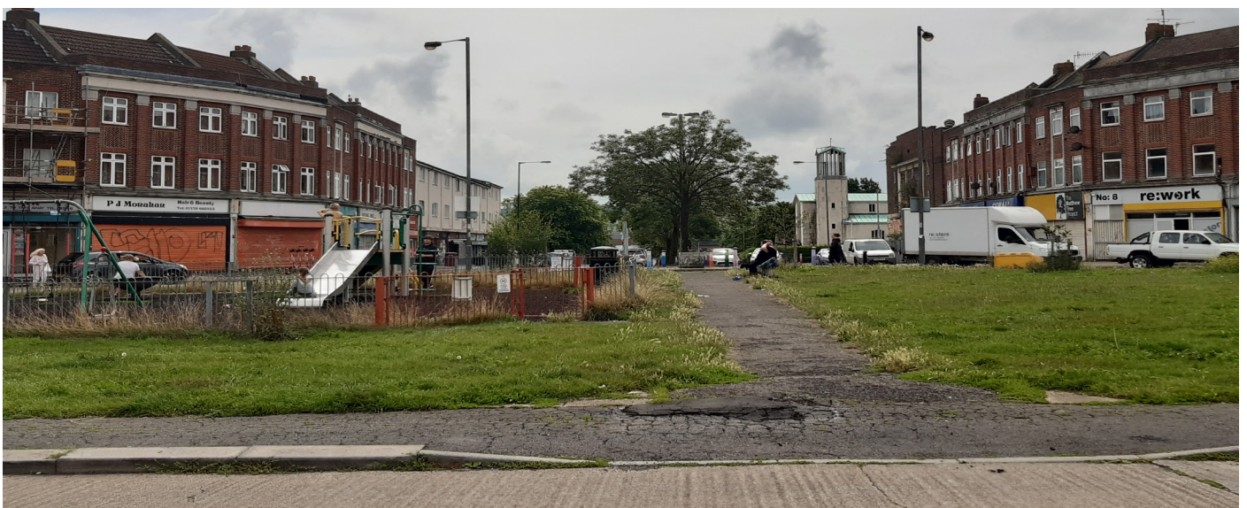
The asphalt walkways around 'The Chase' Green are damaged, unattractive, and potentially dangerous
