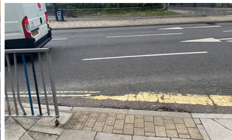
Tactiles indicate crossing where no crossing exists
